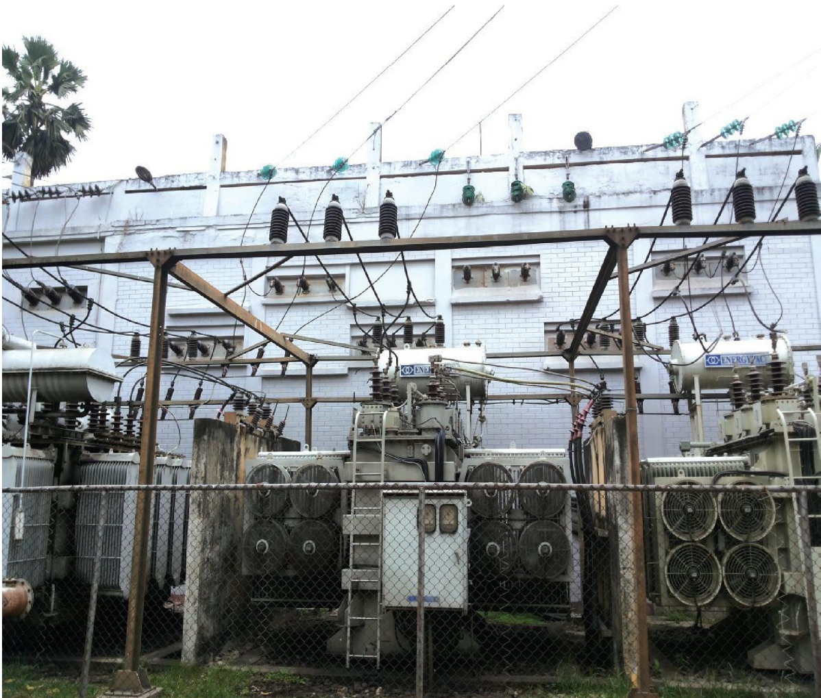
Power Transformers at Joragate 33/11 KV Substation.
